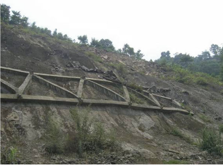
Fig. 2.14 Post-quake appearance of slope surface reinforced by RC frame
