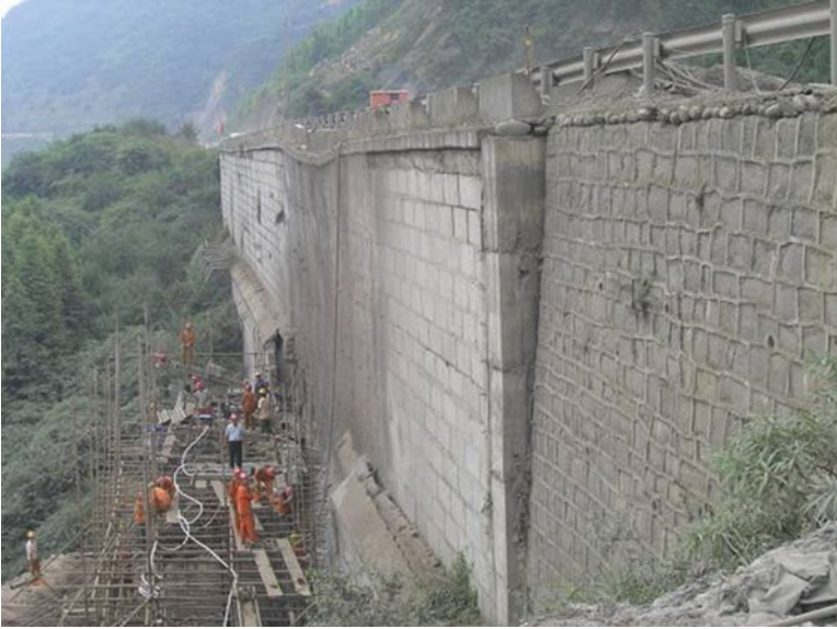
Fig. 2.16 Post-quake appearance of reinforced embankment
