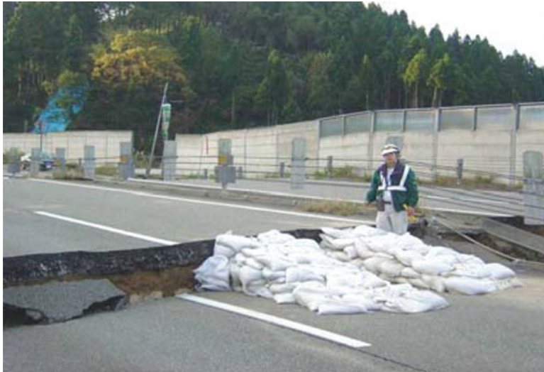
Photo 9.5 Differential settlement between embankment and culvert at C-Box Kawaguchi 11
