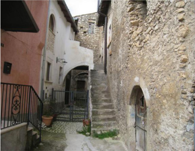
Fig. 1.51 Typical unreinforced masonry structures in the village of San Pio delle Camere suffered no damage (D0), or slight cracking (D1). Structures in this village are similar to those in Castelnuovo
