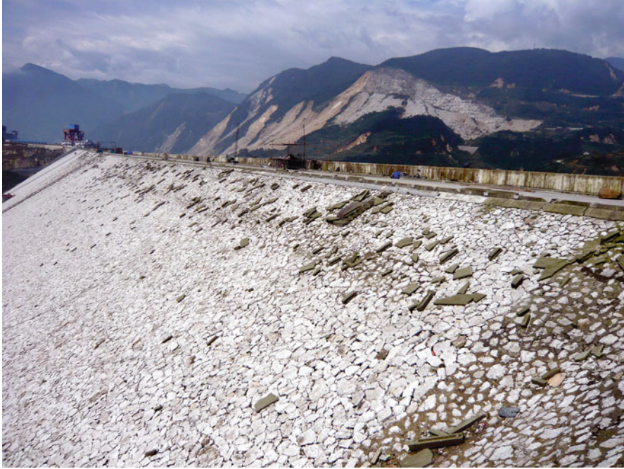
Fig. 10.19 Damage to parapet wall
