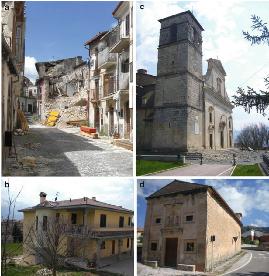
Fig. 1.54 Poggio Picenze: (a) variable damage (D3-D4) on masonry buildings of different style, (b) undamaged r.c. house (D0) close to the (c) monumental church (D3); (d) D1 damage in a church built on coarse-grained Pleistocene formation
