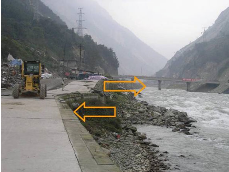
Fig. 2.28 Fault-induced damage in retaining wall in Yingxiu
