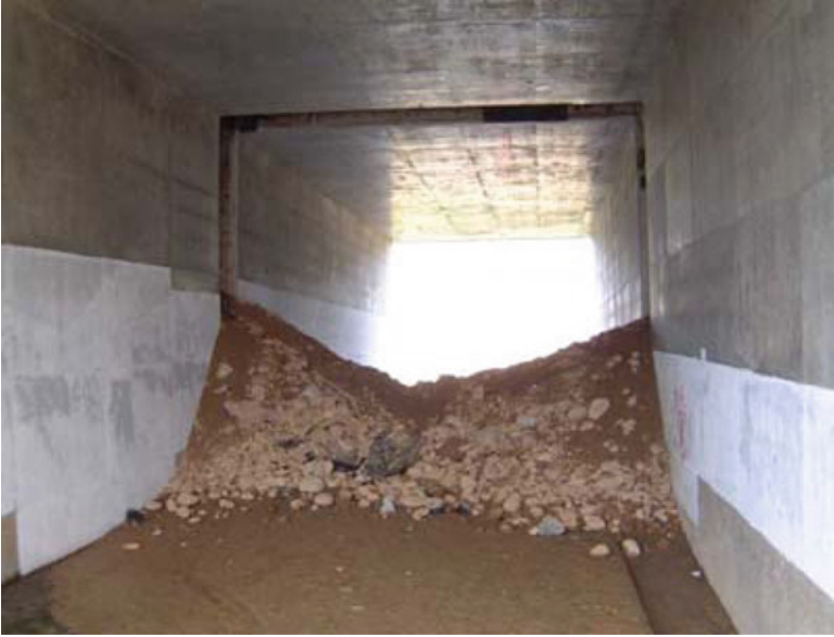
Photo 9.8 Separation of culvert joint at C-Box Ojiya 2
