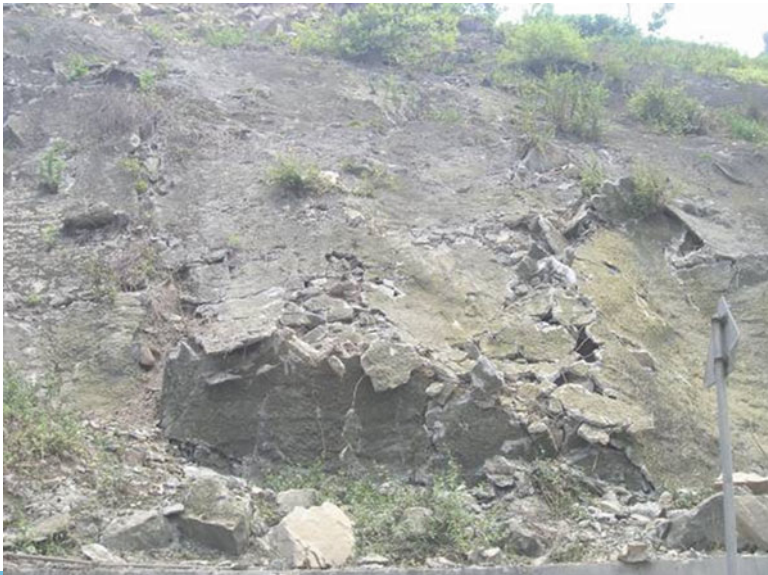
Fig. 2.13 Post-quake appearance of rock slope reinforced by shot crete and metal fence
