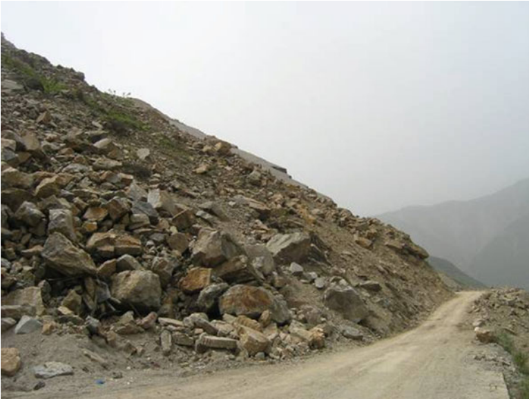
Fig. 2.12 Failure in a slope with geological stratification parallel to surface.
