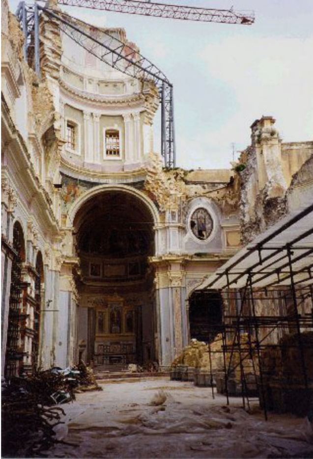
Fig. 8.1 The collapse of the main and right naves and of the dome after the damage caused by the 1990 South-East Sicilian earthquake
