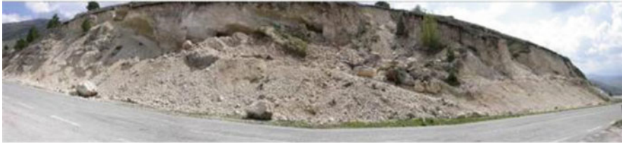
Fig. 1.59 Slump along the road from Barisciano to S. Stefano (Photo by D. Calcaterra and M. Ramondini, University of Naples)
