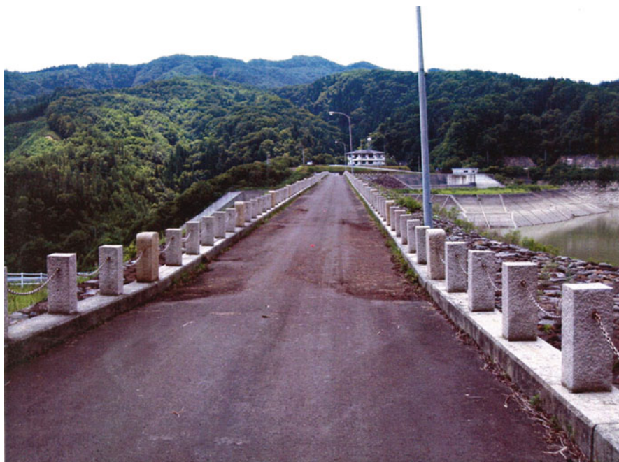
Fig. 10.13 Crest of the Aratozawa dam after the earthquake
