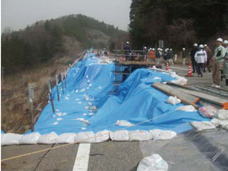
Photo 9.2 Slide of the embankment of Noto-yuryo road at site No.9
