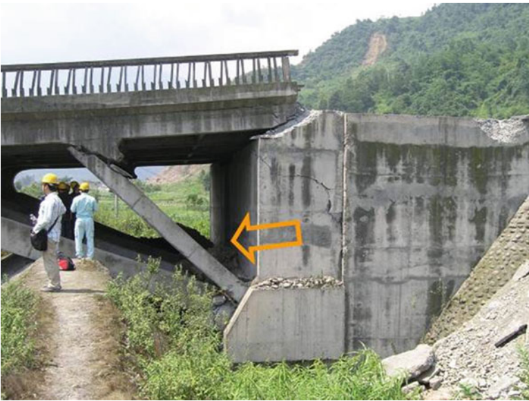
Fig. 2.25 Seismic displacement of abutment of Xiaoyudong bridge
