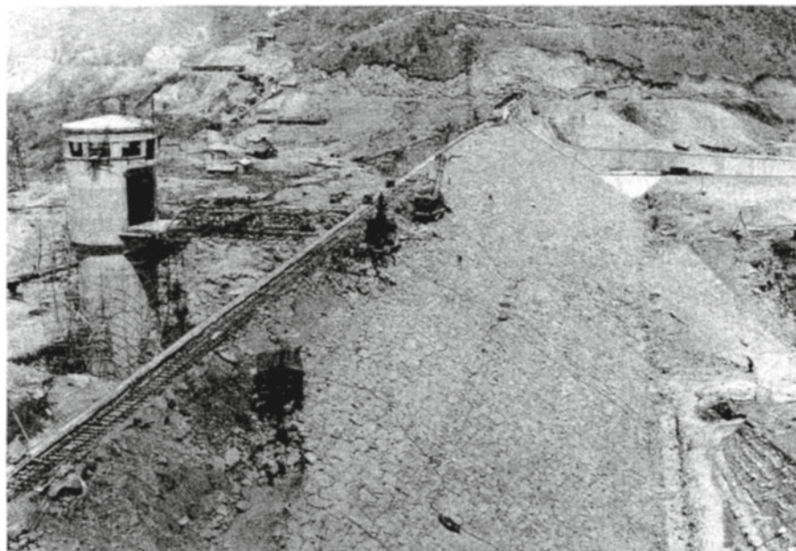
Fig. 10.7 Cranes placing surface rocks near completion of Ishibuchi dam (From the office of Ishibuchi dam)
