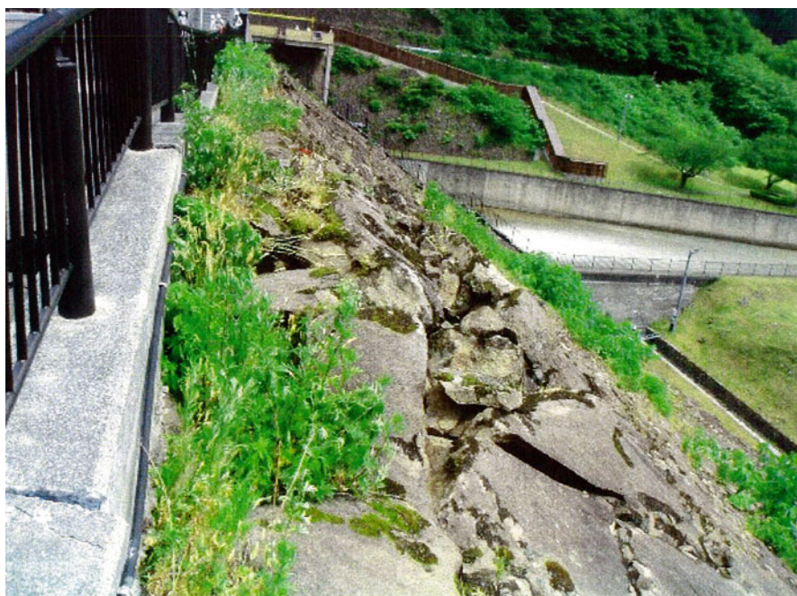
Fig. 10.9 Stone face bulging out near the downstream crest, Ishibuchi dam (Looking towards the left abutment)
