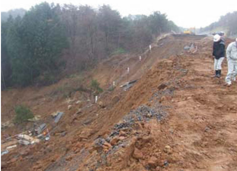
Photo 9.3 Slide of the embankment of Noto-yuryo road at site No.32
