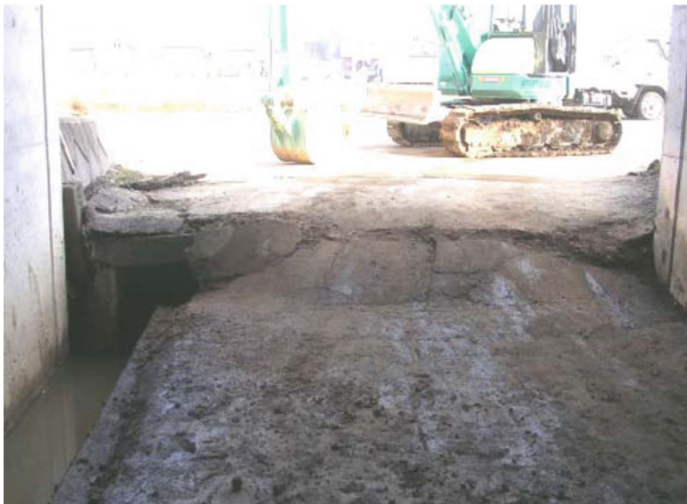
Photo 9.7 Settlement of culvert at C-Box Kawaguchi 22
