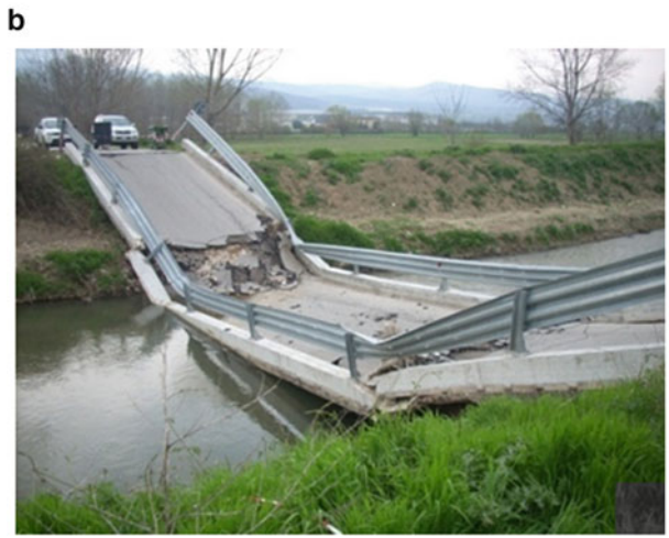
Fig. 1.23 (a) Stratigraphic logs and profiles of the cone penetration resistance q_c obtained from boreholes and CPT tests executed on the two banks of the Aterno River after the April 6, 2009 earthquake in correspondence of the collapsed bridge (b) on the road to Fossa
