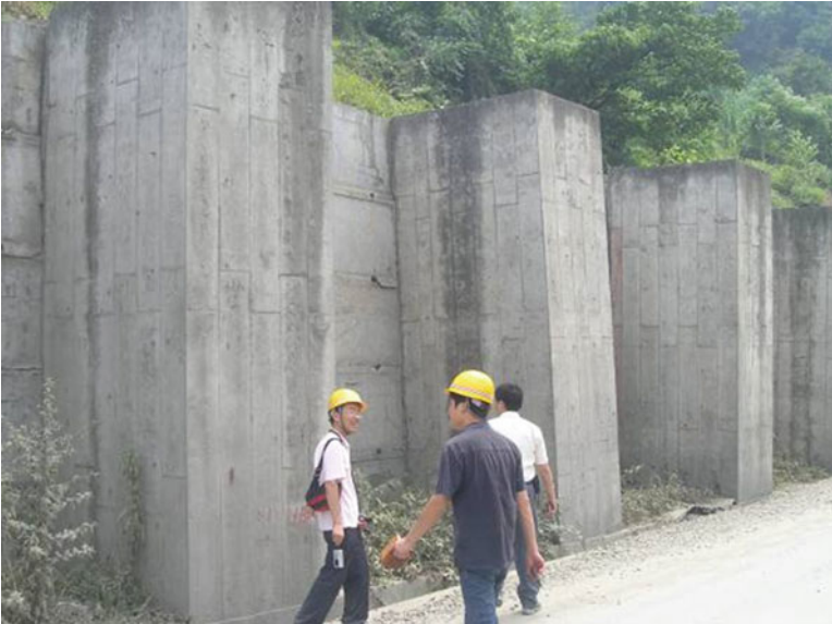
Fig. 2.15 Post-quake appearance of slope that was stabilized by bored piles and panels
