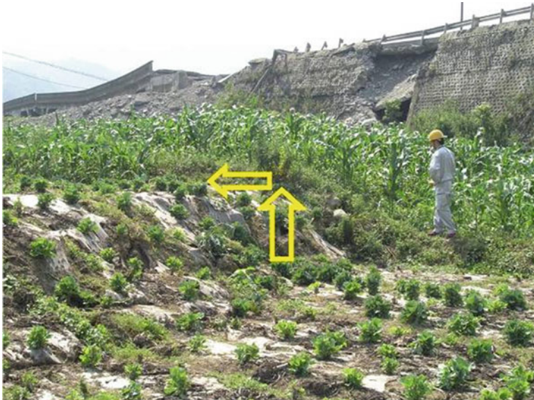
Fig. 2.27 Fault-induced damage in road embankment and stone wall
